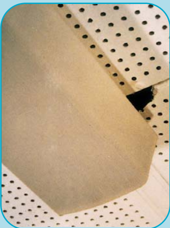
Perforated AIB ceiling tiles
