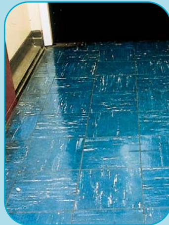
Asbestos-containing floor tiles
